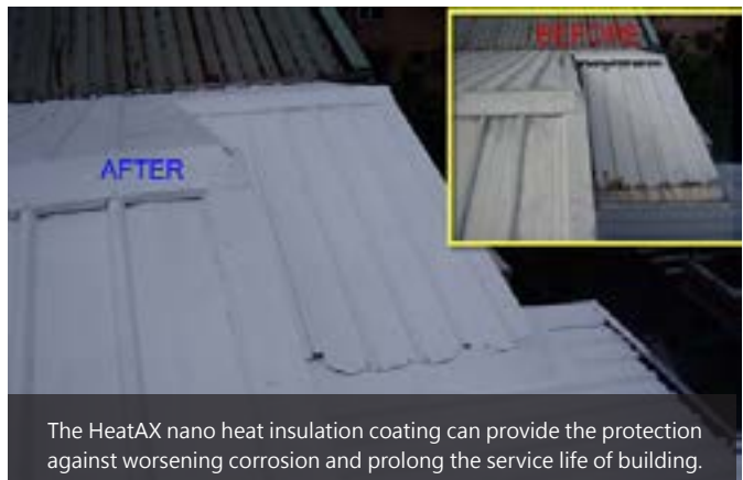
For the corroded sheet iron, the rust removal and patching treatment will be applied first.
